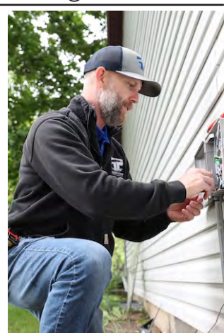
Fiber Technician Matt Jay brings the fiber cable into subscriber's home.
