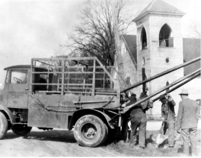
May 1936: Rural electrification begins when articles of incorporation are signed for Paulding Putnam Electric Co-operative. The first pole was set less than two years later. At right is Guy Bidlack, one of the incorporators.
