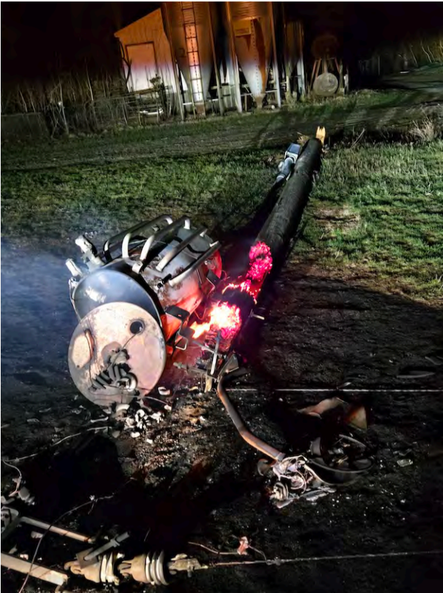
Transformers are not impervious to wind and storms. This one caught fire and burned the pole as power shorted from damage.
