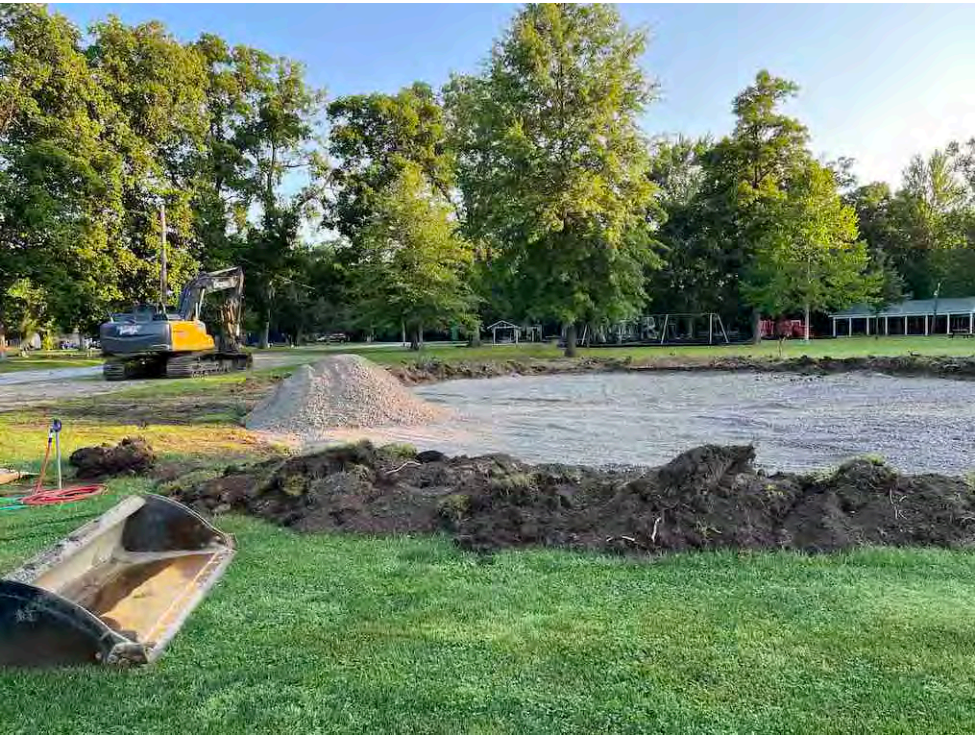
Ben Kauser Excavating broke the ground for Holly Beach Splash Pad this past week! Stay tuned for additional updates about this community project. Follow Holly Beach Splash Pad on Facebook for more information.
