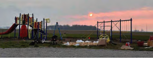
Construction is underway for the new Kiwanis playground at Lela McGuire Jeffery Park in Paulding.
