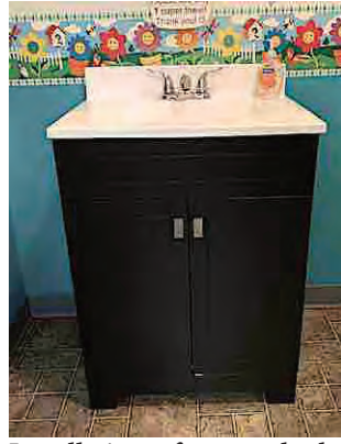
Installation of a new bathroom sink for the littles at Ann's Bright Beginnings by My Father's Hands Handyman Services.
