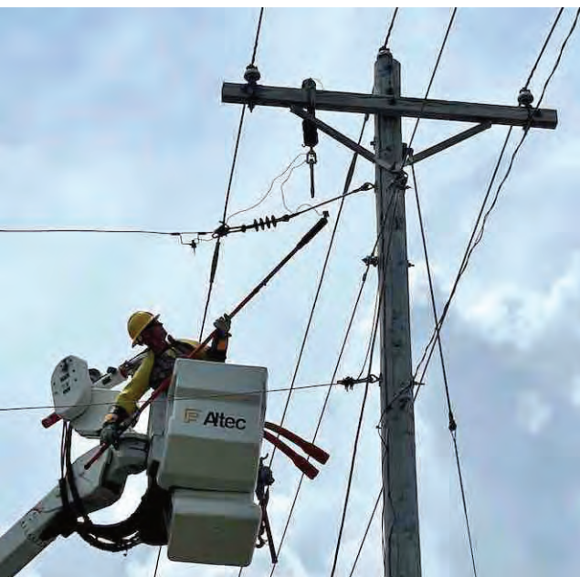
PPEC Lineman Brandon Burelison works on a power line. PPEC introduces their new right-of-way tree-trimming and vegetation management contractor, Mint City Utility Services, who will begin work this month.
