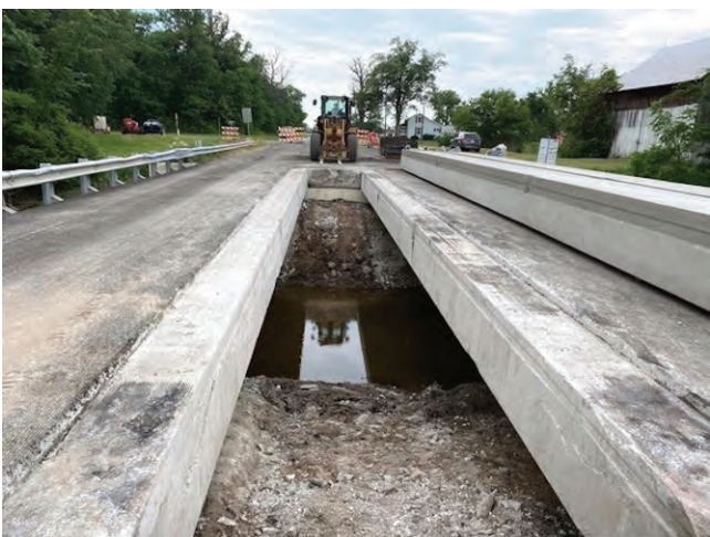
The large opening in the U.S. 127 bridge over Lost Creek in Defiance County where a deck replacement project is now delayed two to four weeks.
