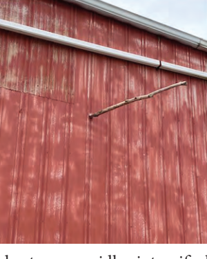
derstorm rapidly intensified as it moved out of southeastern Allen County, Indiana into southwestern Paulding County. Damaging winds, ranging between 60 to locally over 80 mph, caused damage from Payne, OH through Latty and south of Melrose. The most extensive damage appears to have occurred from Payne to Latty where tree damage, minor structure damage and damage to power poles occurred. Tree limbs also fell onto parked vehicles, causing damage. A resident shared a picture on the Paulding County EMA Facebook page, south of Latty showing a home weather station recorded an 83.4 mph wind gust. We would like to thank
