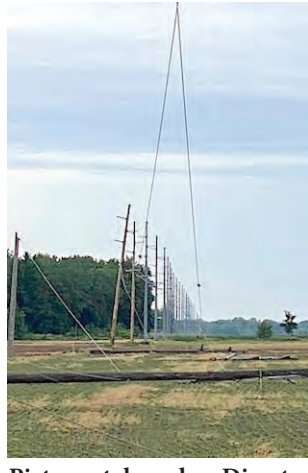
Picture taken by Director McCoy shows the damage of the rotating winds at the farm on as well as the straight line winds that took down five power poles.
