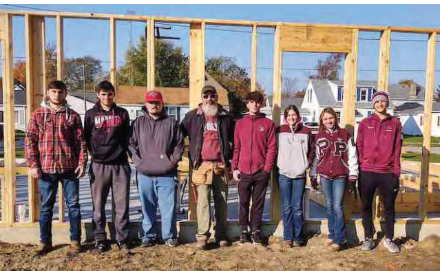
The shop class from Paulding High School putting up the walls for the Habitat house. Left to right: Logan Vance, Dylan Kuckuck, Wyatt Beckman, John Kennedy, Christian Bauer, Alana Eddings, Janae Pease, Nick Manz.
