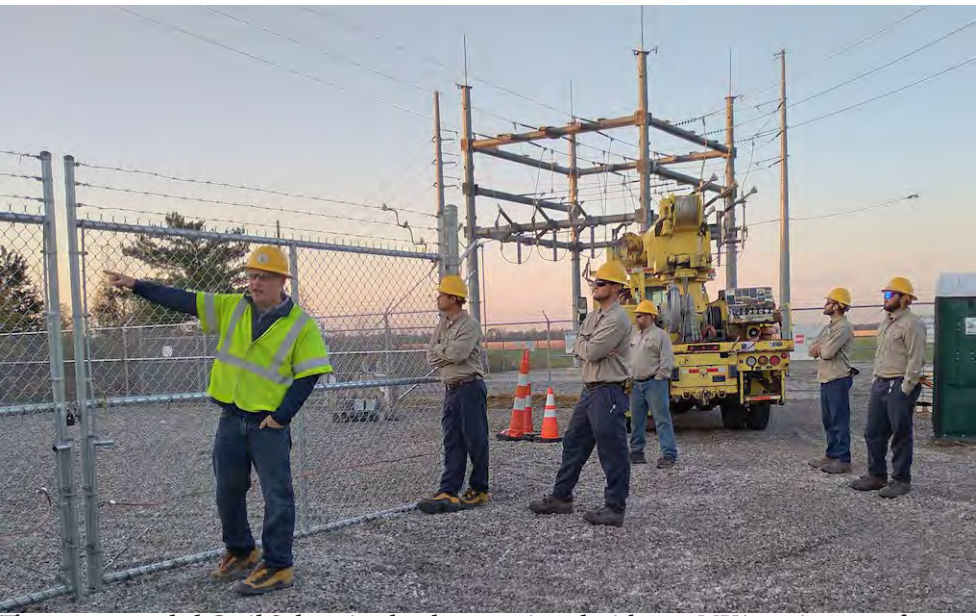
The new, upgraded Cecil Substation has been equipped with a 12 MVA station transformer, more than twice the capacity of the old transformer. (right) PPEC's crews complete a walk-through safety inspection of the new Cecil Substation before being energized.
