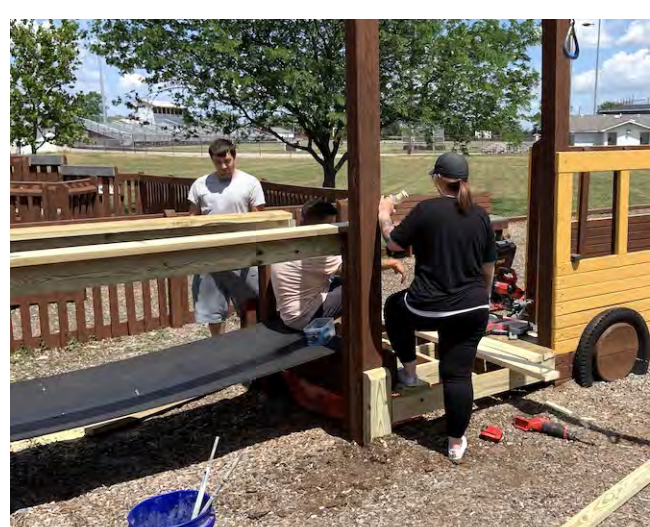
Teamwork and cooperation as well as alot of sweat went into the repairs this past weekend.
