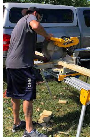
Volunteers brought out their own tools to make the necessary repairs to the playground equipment.
