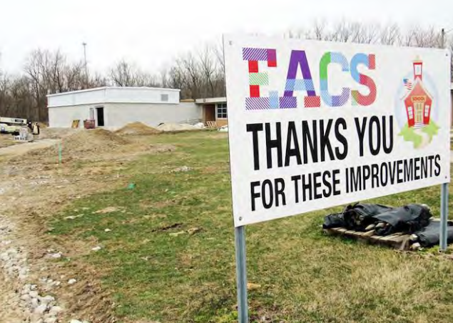
A 3,000 square foot machine shop (background) is being added to the East Allen Career Center in the former Meadowbrook Elementary School and former New Haven Intermediate School. It will house the precision machining workshop and begin operating in the fall of 2020. It is one of six programs available to juniors and seniors in the five East Allen Schools high schools. Photo by Rod King.
