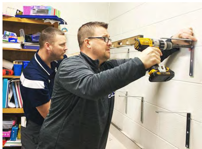
Antwerp teachers, Mr. Messman and Mr. Hoepfner, install some shelving in classrooms during the pandemic school closure. Photo via Antwerp Local School Facebook page.
