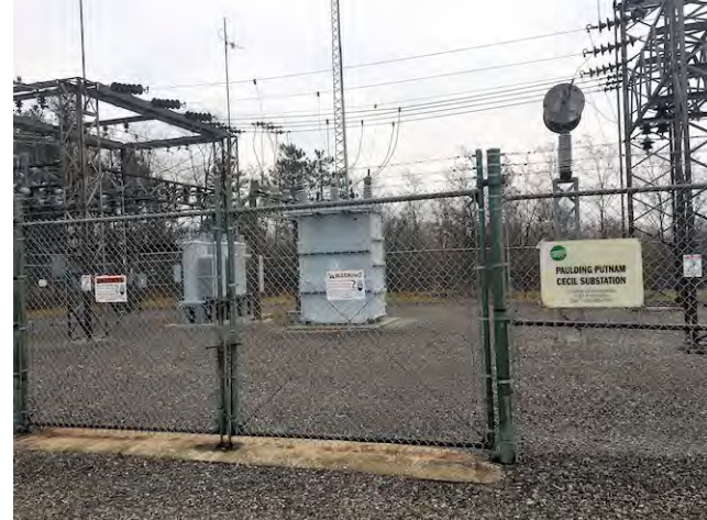
PPEC's Cecil Substation is slated for a rebuild in 2020 to improve electric reliability, system durability, and increased load capacity for PPEC members.
