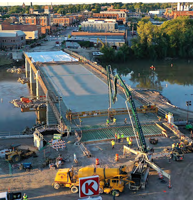
By 8:00 a.m. the work is nearly completed as there are only a few feet to go. The concrete is then being covered to protect it while it cures.
