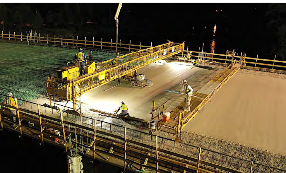
At 9:00 p.m. it appears that the work is about 20% done being poured, starting on the south end.
