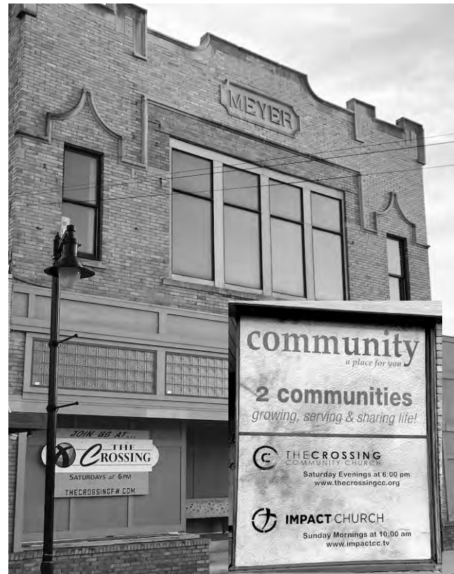
The installation of the vinyl is just finished as the storefront building is cleaned up from the ladders and tools needed to finish.
