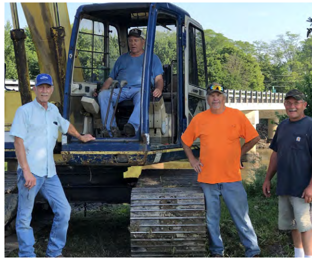
We are preparing Cecil Bridge river access for a stoned parking lot is being prepared. Drive by and see the new improvements. Pictured is Tim Franklin, Jim Pendergrast, Gary Mabis and Brad Dysinger. Your hard work is appreciated.
