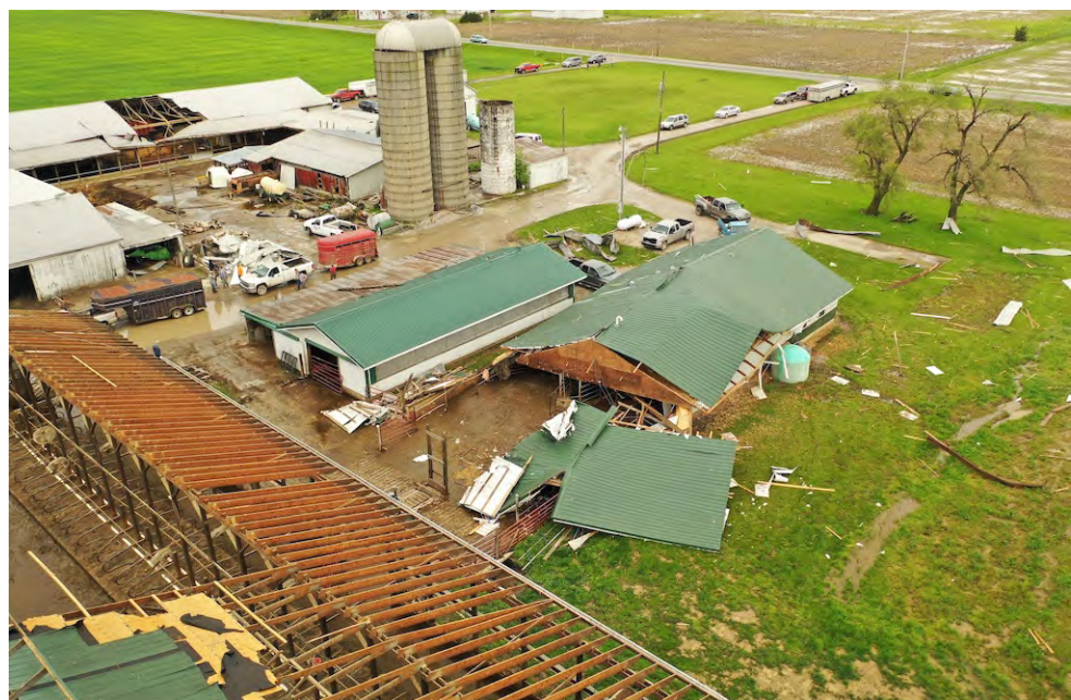
The Schlatter Dairy Farm on SR 111 was hit by a major storm on Thursday morning, causing heavy damage to the buildings on the site.
