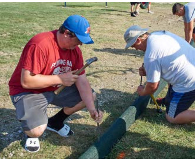
Jacob Stouffer and Matthew Stouffer from the Wayne Trace Football team drive in rebar to secure the perimeter.
