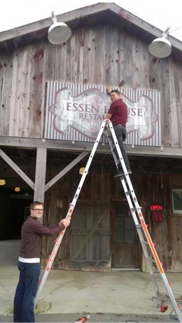
West Bend employees work to install the new sign at the restaurant on Friday evening.
