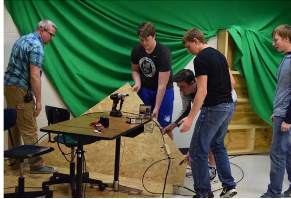
Mr. Cord Ehrhart helps EYF students Houston Mansfield, Cole Seslar, Dalton Foreman, and Seth Rister put together flooring for the new broadcast set.
