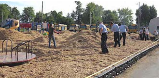
Vantage Building and Grounds students, along with their teacher Dave DeLano and teacher's aide Brenda Wurst, pitch in to level the huge piles of mulch at the Payne Elementary School Playground Project.
