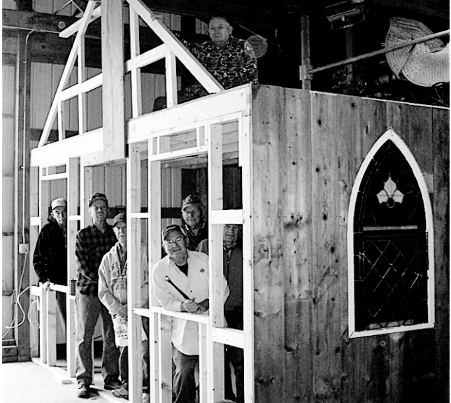
JPHS men volunteers are building a Chapel in Barn One at the museum. Pictured from left to right: Dave Stouffer, Denny Sanderson, Roger Sierer, Bill Strahley, Max Kochensparger, John Pier and up on the roof is Dan Wilder.
