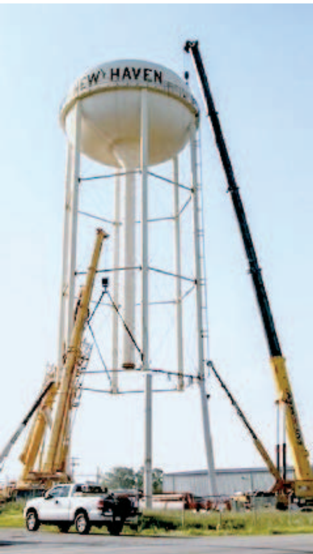
Wessler Engineering Ryan Road water storage worked with the City of New Haven, Indiana on a tank raising project at their tank.
