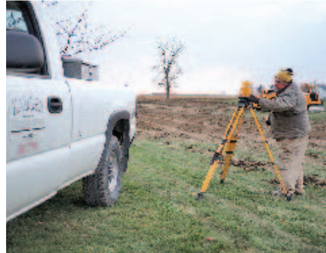
Walt Kauser of Kauser Excavating is surveying after moving dirt around in preparation for the new baseball diamond.
