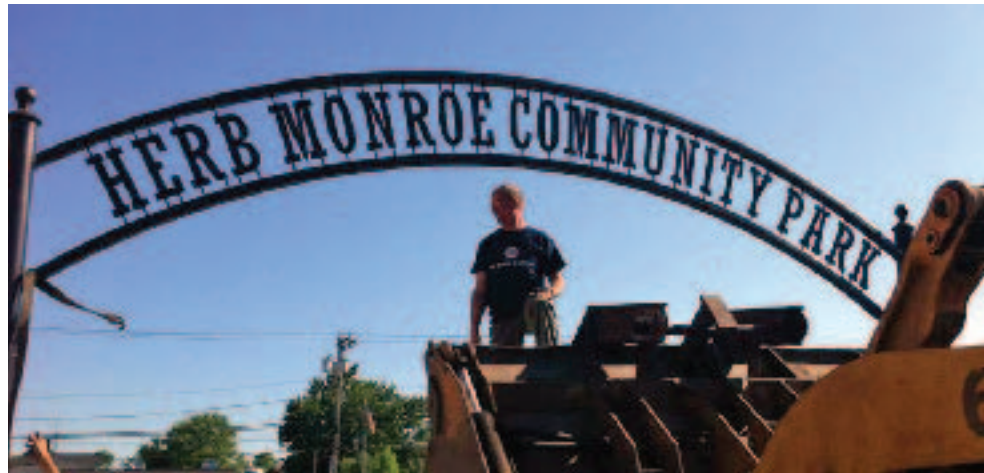
Mark Greenwood, designer and builder of the new Herb Monroe sign, guides the iron structure as it's being set in place at the new park on Tuesday, June 9th. Photo by Erika Willitzer.
