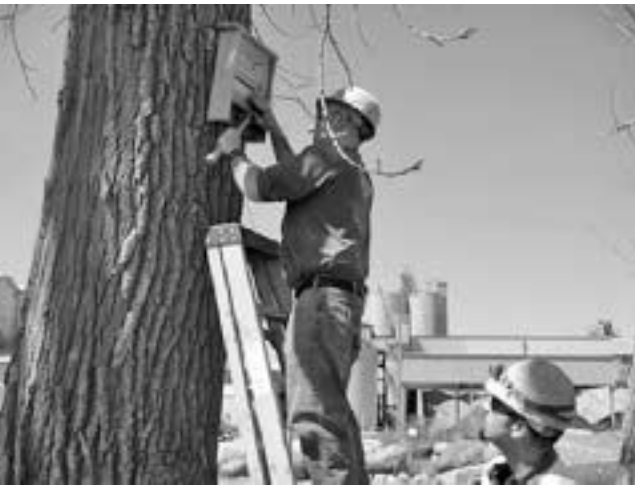
Lafarge Paulding employees, Tracy Smith (left) and Ben Johnson (right), install the site's new bat shelter.
