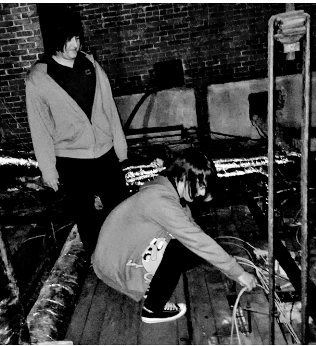
Vantage Network Systems seniors Wyatt Sawyer (Paulding) (left) and Dylan Boroff (Lincolnview) check out the network cables in the attic of the Van Wert County Courthouse.
