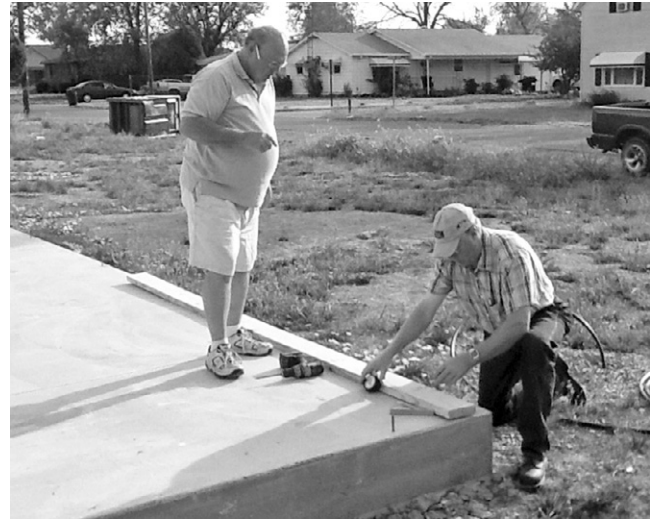
Habitat members, Keith Klopfenstein and Al Lininger are shown preparing to start the next Habitat home.
