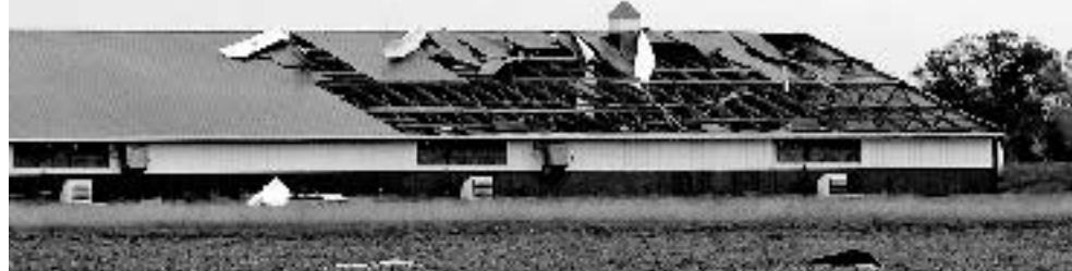
Klopfenstein Family Swine Farm - storm damage
