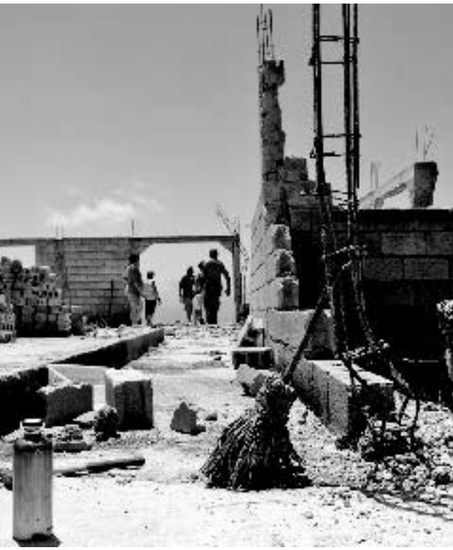
A Grace Gathering mission group works to clear away the rubble of what used to be a school at an orphanage in Calebasse, Haiti. This is what remains of the second story of the school after the earthquake in 2010.
