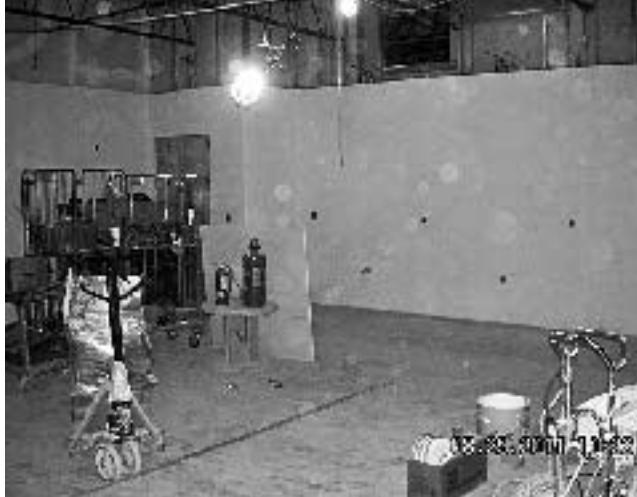
Concrete block walls are up, drywall is being hung and additional work continues in one of the new high school Health Technology labs at Vantage.
