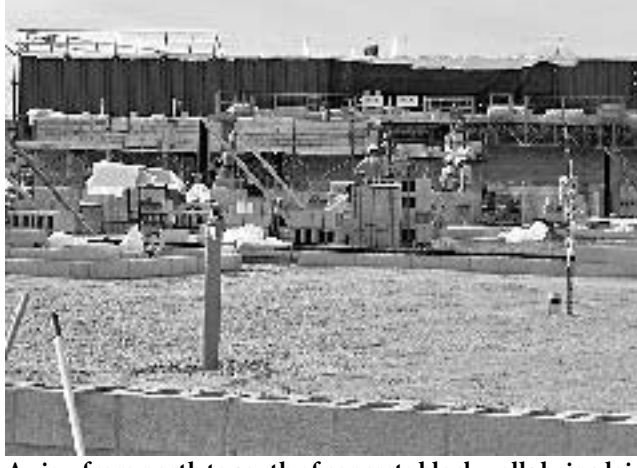
A view from north to south of concrete block walls being laid and other work on the new addition to Vantage.
