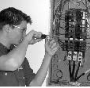
Christ Stalsberg, a senior Electricity student from Wayne Trace, installs a breaker in the panel at the YWCA.
