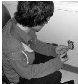
Vantage's Tony Valle (Paulding) installs a receptacle outlet in the fitness center at the YWCA.
