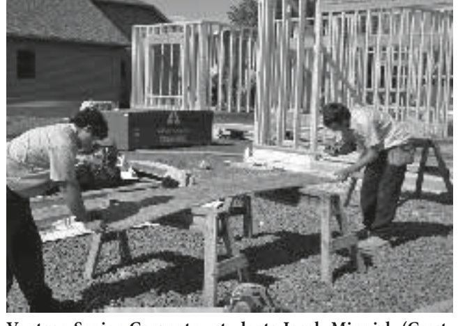
Vantage Senior Carpentry students Jacob Minnick (Crestview) and Rich Klinger (Crestview) are snapping a chalkline for exterior wall sheathing for this year's house, located in the Washington Place subdivision in Van Wert.
