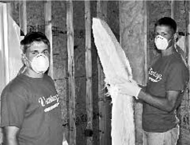
Vantage Student Ambassador Todd Akom (Wayne Trace) and Brian Voisard, Jr. (Van Wert) install insulation at this year's Habitat for Humanity House on the Day of Caring.
