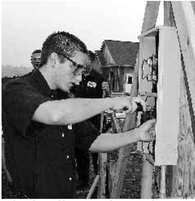
Cody Fitch, a Paulding senior in the Vantage Electricity program, works on the temporary electrical service at this year's construction house project in the Washington Place subdivision in Van Wert.
