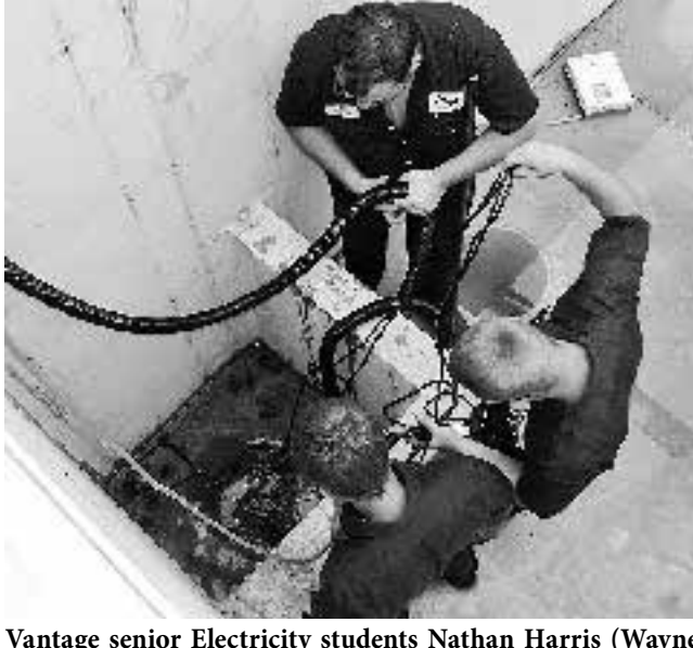
Vantage senior Electricity students Nathan Harris (Wayne Trace), Gunther Mohr (Crestview) and Jesse Barker (Lincolnview) check out the sump pump installation at the construction house project.
