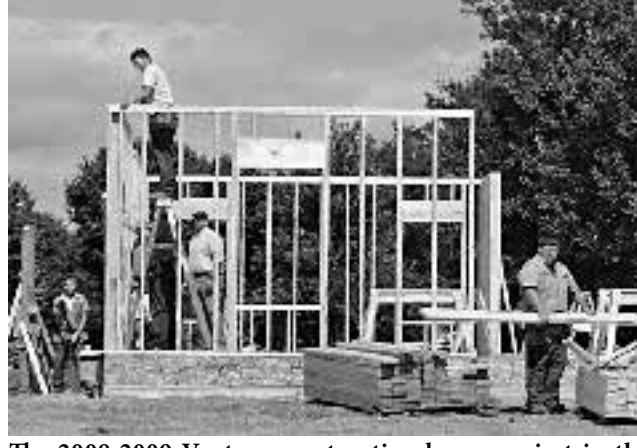
The 2008-2009 Vantage construction house project in the Washington Place subdivision in Van Wert begins to take shape.
