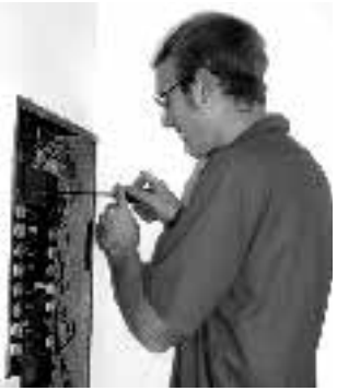
Vantage Electricity senior Eric Beck from Paulding works on the fuse box at the new offices of the Van Wert Visitors and Convention Bureau and Main Street Van Wert.
