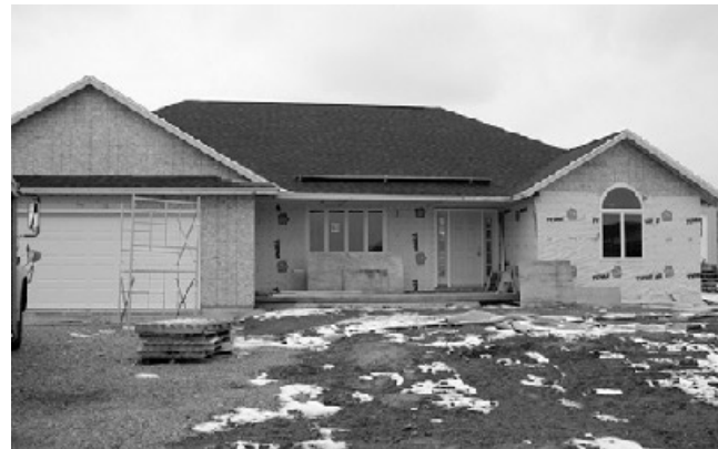
The 2006 Vantage Career Center construction house project on Bruns Avenue in the Washington Place subdivision.
