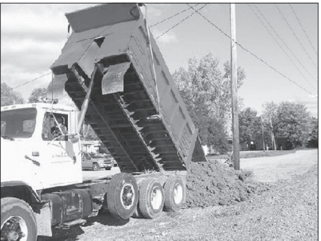
Kauser Trucking unloading dirt at the beautification project east of Antwerp. Kauser's donated the truck and driver at no charge. Thanks Kausers!
